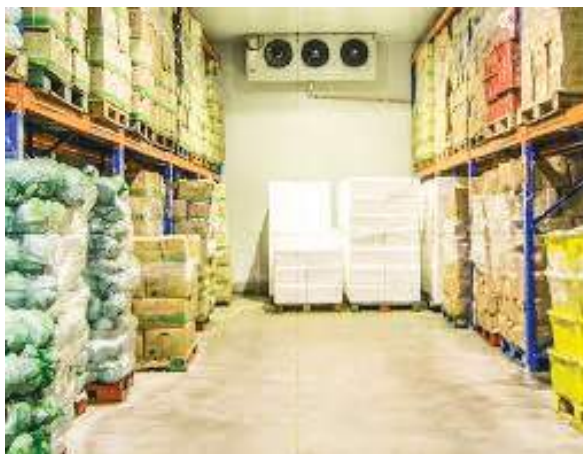
Figure 1.38 Cold Chain Storage
